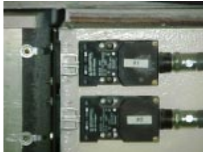
Figure 3: Shield door interlock switches are shown. The mounting is positive-mode, whereby the keys that engage the switch move with the door. Each switch has two redundant contacts. The safety processor monitors pulse trains that travel through the cable and contacts, enabling discovery of both open and short failure modes..
