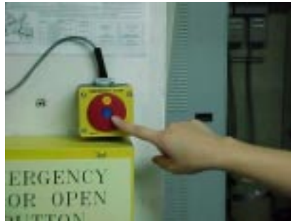
Figure 1: Emergency-stop buttons are placed at the exits of all shielded vaults.
