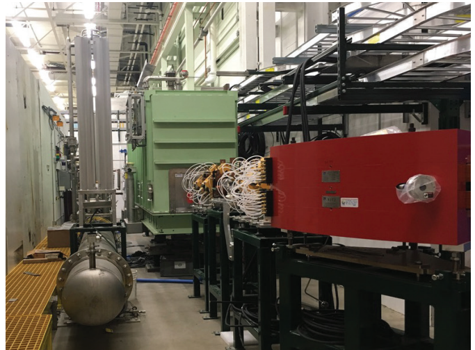
View of the ReA6 cryomodule and new high energy beam line in the ReA6 accelerator vault.
